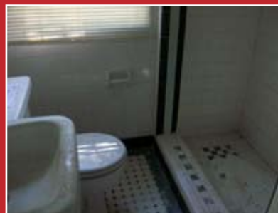
Bath in Basement
